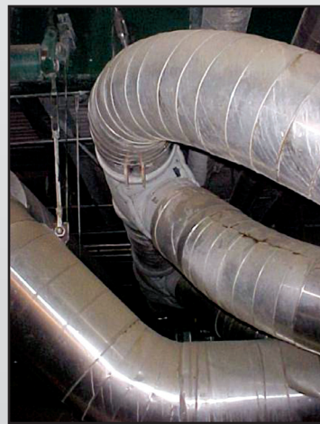
Main Steam System with Support Problems.
