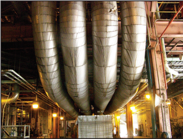
Bottom of the vertical run, Hot Reheat and Cold Reheat lines.
