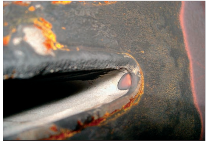
Figure 9: Through-wall penetration of the tube wall immediately below the seal weld at the tube entry. Also note the loss in material of the seal weld. This is recorded as DHACI 5.
