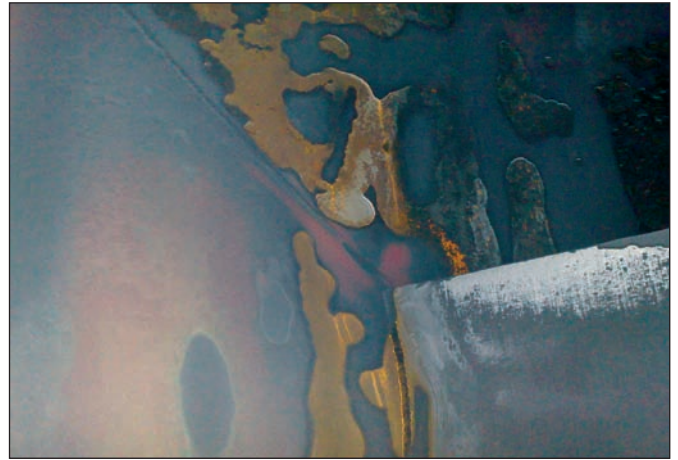
Figure 12: Localized area of significant wall loss in the lower exhaust duct. DHACI C.
