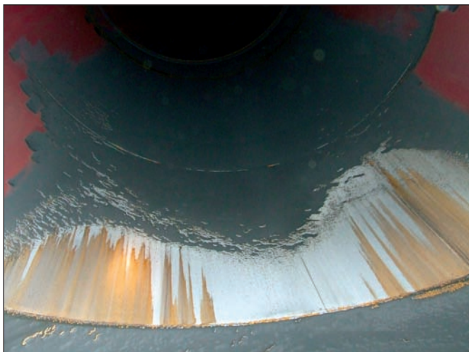
Figure 14: Corrosion pattern in branch H2-V3 (Figure 7). DHACI C.
