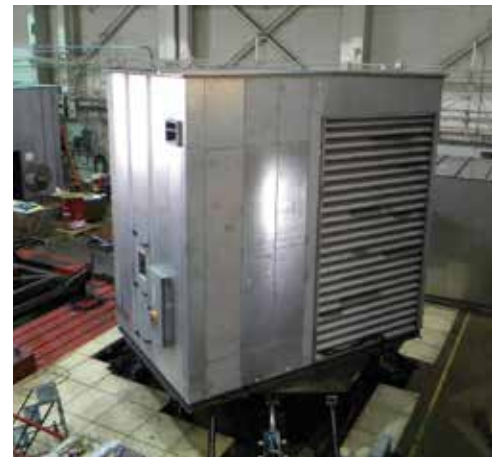
Air Handling Unit Awaiting Seismic Testing
