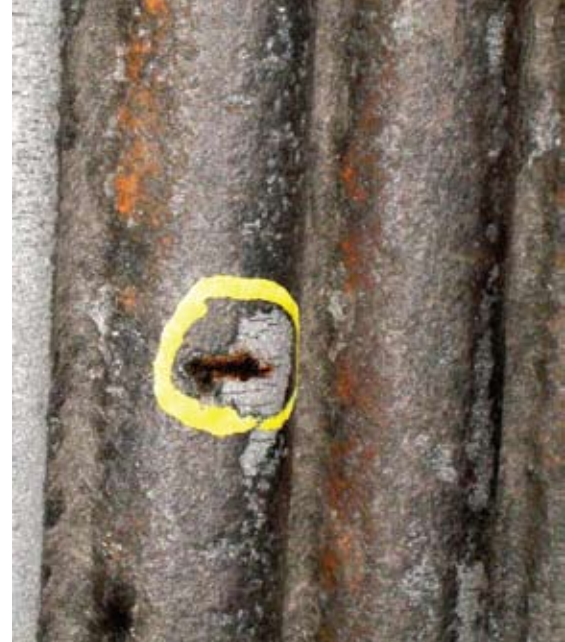
Figure 1 Overall view of the leak of Front Wall tube 124 noted during the field examinations on May 15, 2009.
