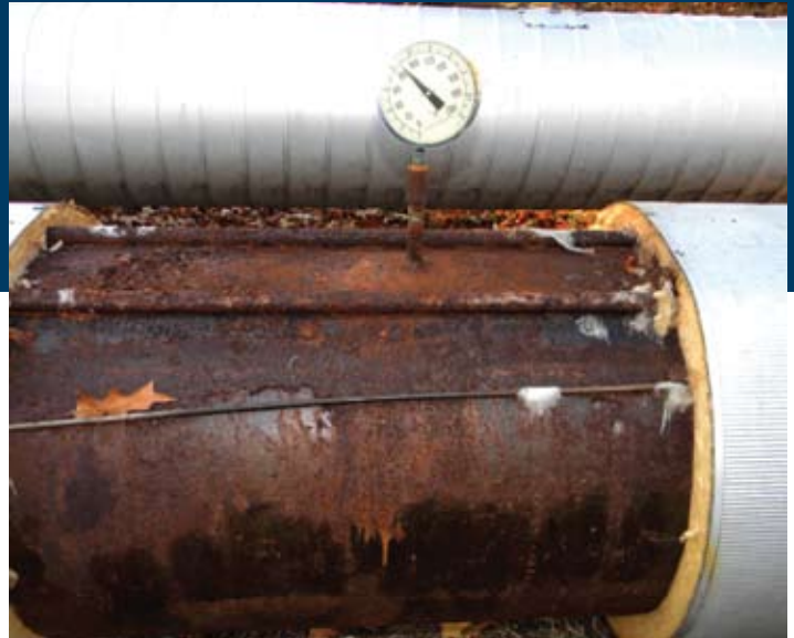
Figure 3. Piping Region Susceptible to Corrosion
