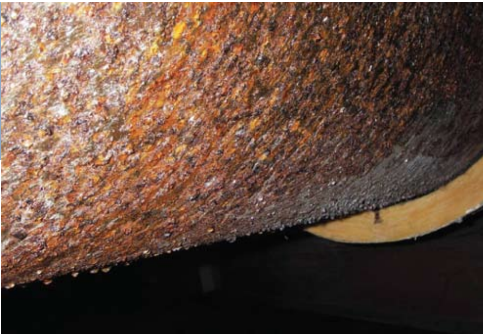
Figure 2: External corrosion on chilled water system
