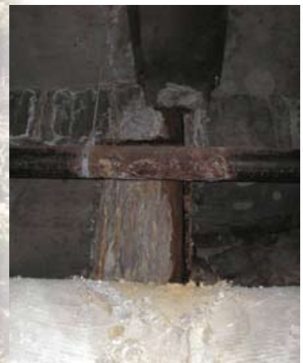
Figure 1: Photo showing area with water dripping from above in tunnel
