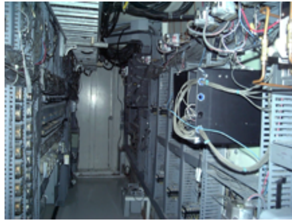
FIGURE 2. Condensate Demineralizer Panel at a BVVR (Inside View)
