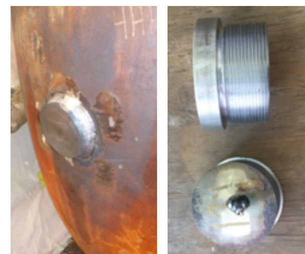
FIGURE 2. Core removal and pipe plugging process. Core Drilling TOP Pipe Spool with Plug Installed BOTTOM LEFT BOTTOM RIGHT Extracted Core LOWER and Replacement Plug UPPER
