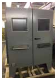
Main HMI Panel
