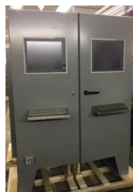
Main HMI Panel
