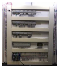
Remote I/O Panel
