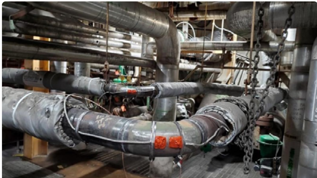
FIGURE 4. Photograph showing Structural Integrity's thick-film ultrasonic sensor technology installed on two high-temperature piping elbows that are susceptible to thinning from erosion.
