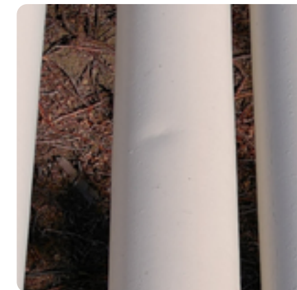
FIGURE 1. Drone image of a dent on an elevated section of pipeline
