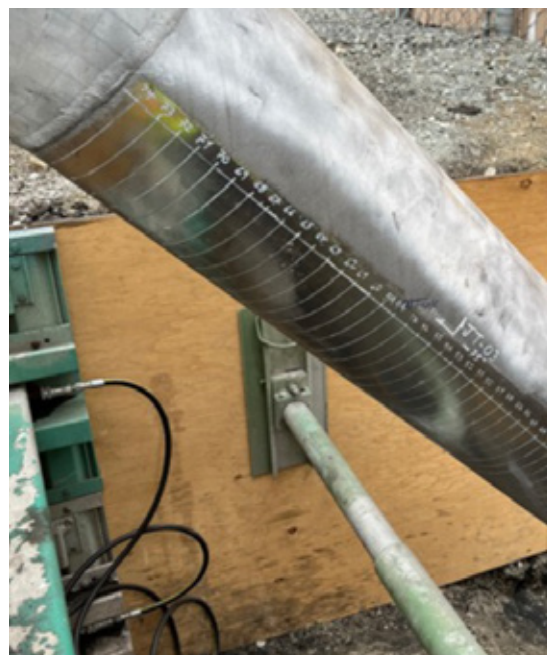
FIGURE 4. Example of facility piping with lap weld inspection applied.
