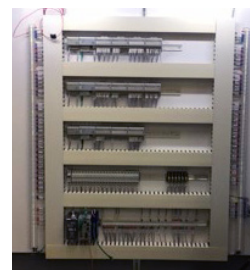
Remote I/O Panel
